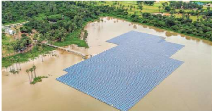
Power on water: An aerial view of the floating solar panels on the Mudasarlova reservoir in Visakhapatnam.
